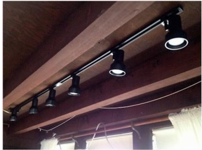
New track lighting
